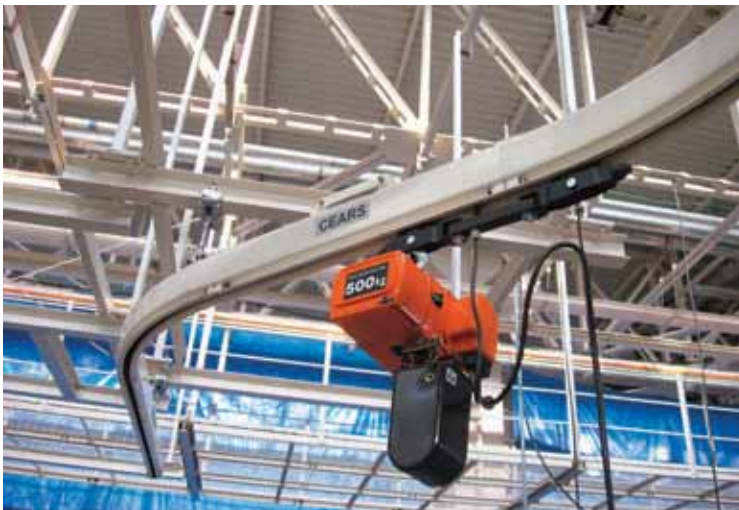
Hitachi Hoists installed on CEARS Rails with Internal Bus Bars
